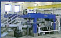
Centrifuges used for dewatering
