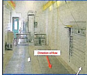
Rack of UV Bulbs
